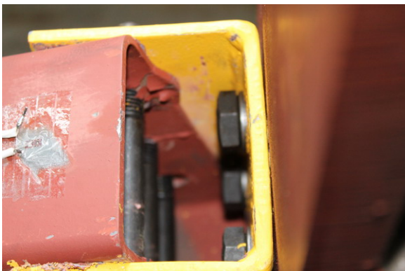
Fig.11 Model SP8/ Collapse of the connection as a result to plastic deformations to cutting the end of the beam in the upper long bolt
